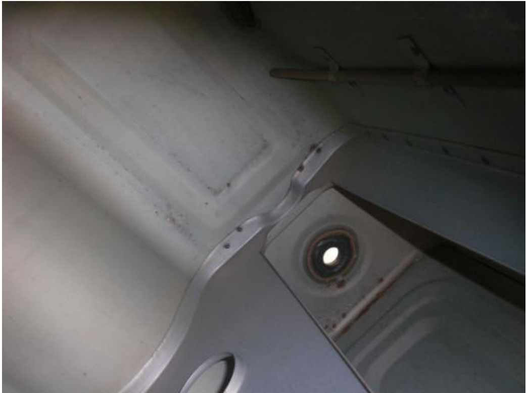
Blasted surface rust off the exterior
